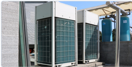
Rooftop VRF Outdoor Condensers
